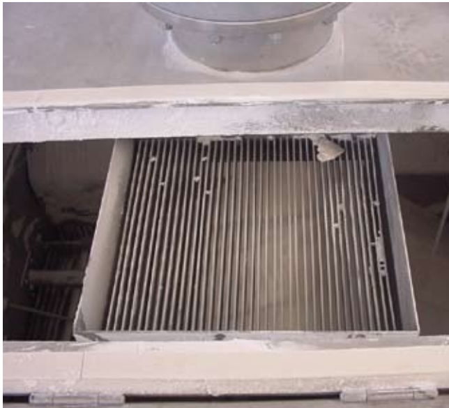
COARSE SCREEN INSIDE INLET HOPPER
