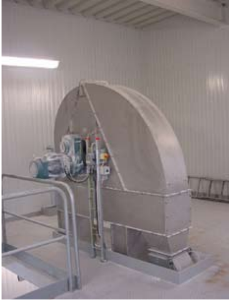
BUCKET ELEVATOR TO TOP OF SOLEX COOLER
