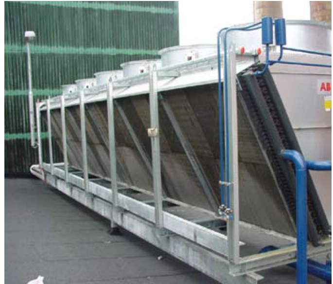
CHILLER FOR COOLING WATER
