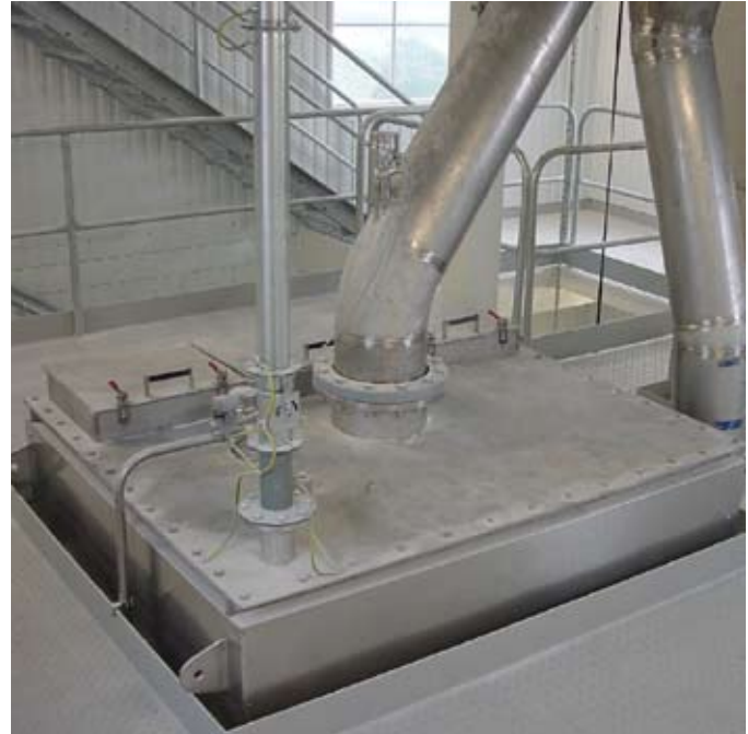
Danisco – Top View of Inlet Hopper
