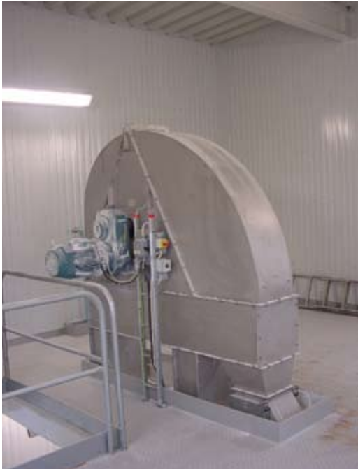
Danisco – Bucket Elevator At Top of Solex Cooler
