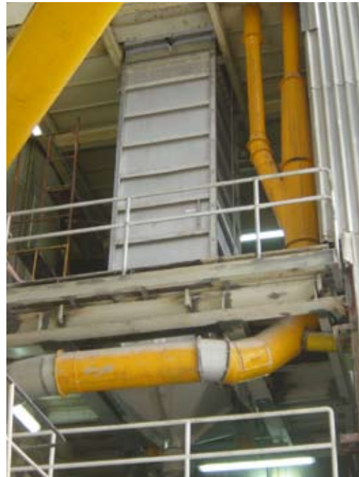
R.A.R – Sugar Cooler and Vibrating Feeder
