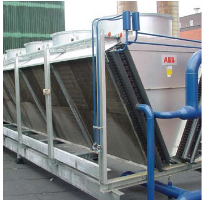
Danisco – Chiller for Cooling Water
